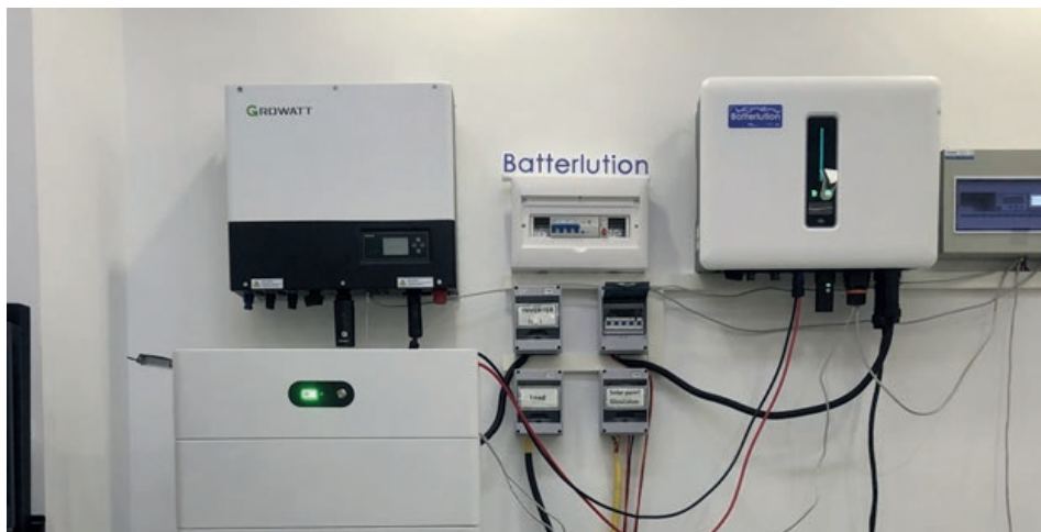
A glowing green residential battery stands to chest height ready to help the grid.
