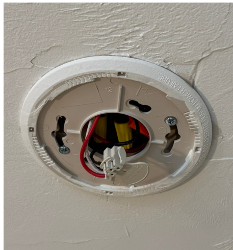
An all-too common sight in rental housing. This puts the lives of other renters at risk.
