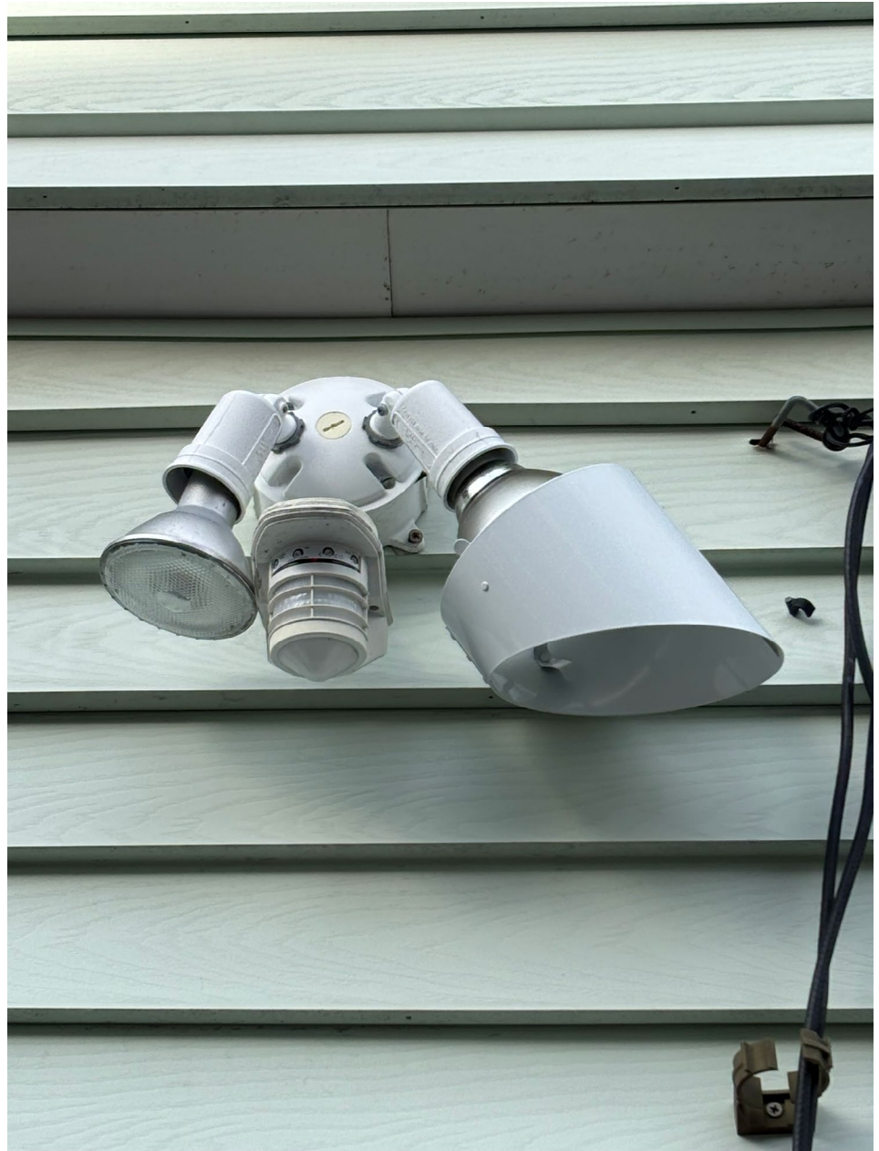
The smaller, unshielded bulb at left produces more light trespass than the larger, brighter shielded PAR-38 at right.
