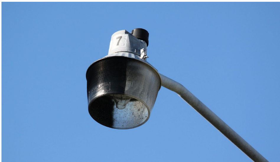
This streetlight is half shielded, fitted with a fully round shield painted black on one side, presumably blocking light trespass toward residents on that side, while scattering light through the glass hood on the other side. Cc by-sa flickr flipfloppflorida
