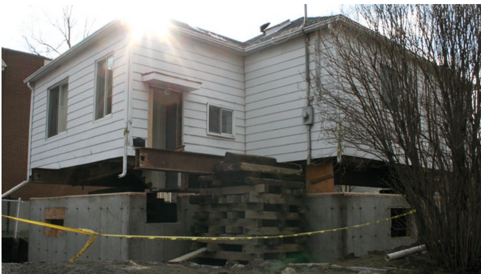
The only solution for a pyrrhotite-damaged foundation is a full replacement. (Image: lic CC BY-2.0 Zanastardust)
