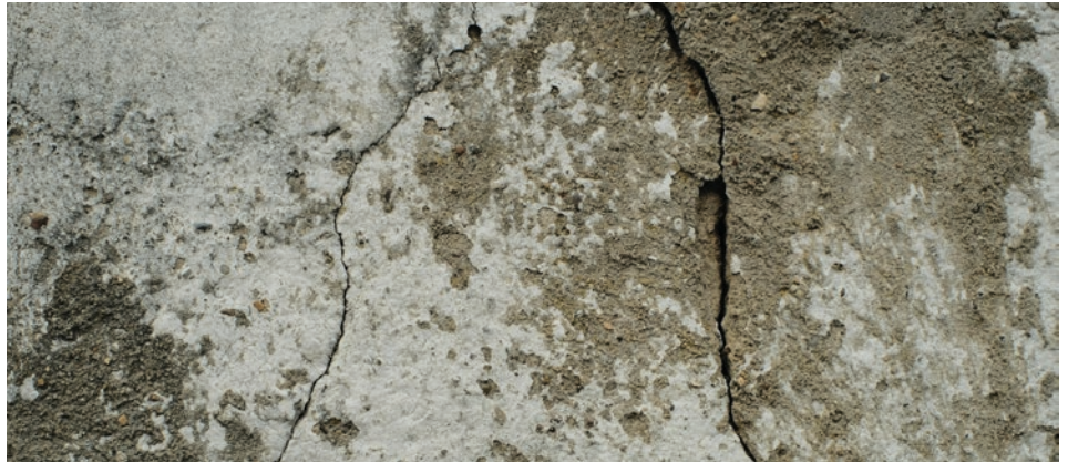
If the cracks in your foundation are from pyrrhotite, then by the time you see them on exterior walls, there's already significant damage. (Image: Rhubbarstockfootage for Unsplash)
