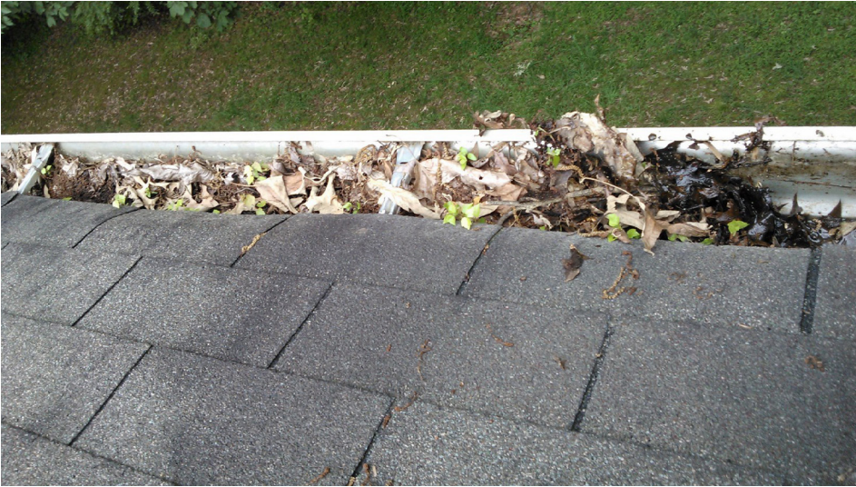
If your gutters look like this, you could use a good handyman. Cleaning overfilled gutters is one of the many odd jobs suited for handyman professionals around homes and rentals. Image: CC BY-SA 3.0 Wikimedia Commons-User:Randall 1022
